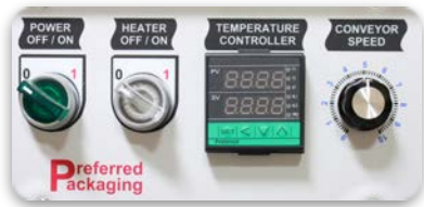
Tunnel Control Panel
